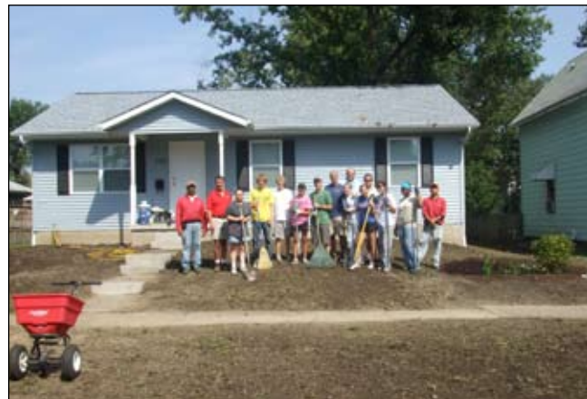
Delf's Landscaping and Aunt Rhodie's Landscaping – two firms from the Quad Cities - along with a group of volunteers, partnered with the Scott SWCD to install three rain gardens and perform soil quality restoration at a new Habitat For Humanities house in Davenport. REAP funding provided financial assistance.
