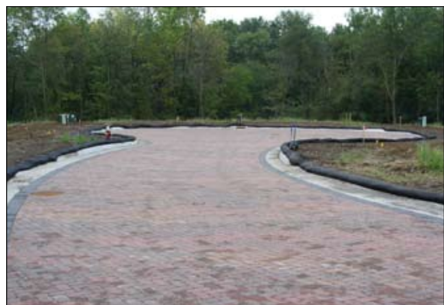
Iowa's first permeable paver street was installed in this Dubuque subdivision in 2009. Stormwater infiltrates through the pavers and is temporarily stored in a rock chamber below ground, which provides water quality protection and eliminated the need for detention basins.
